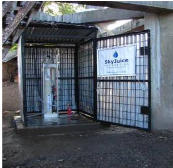
A SkyHydrant™ water filtration system
