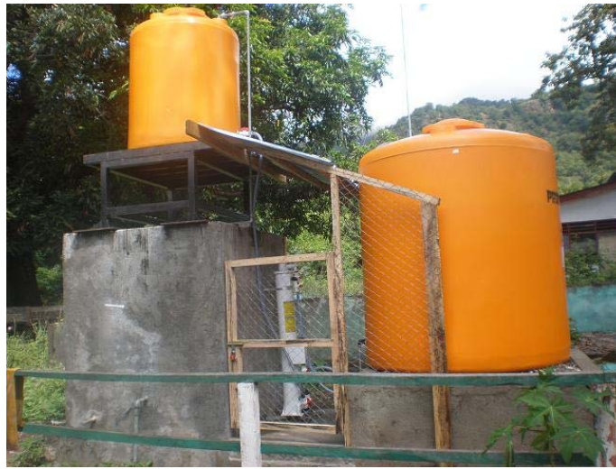
Tank stands and tanks with water filtration unit
