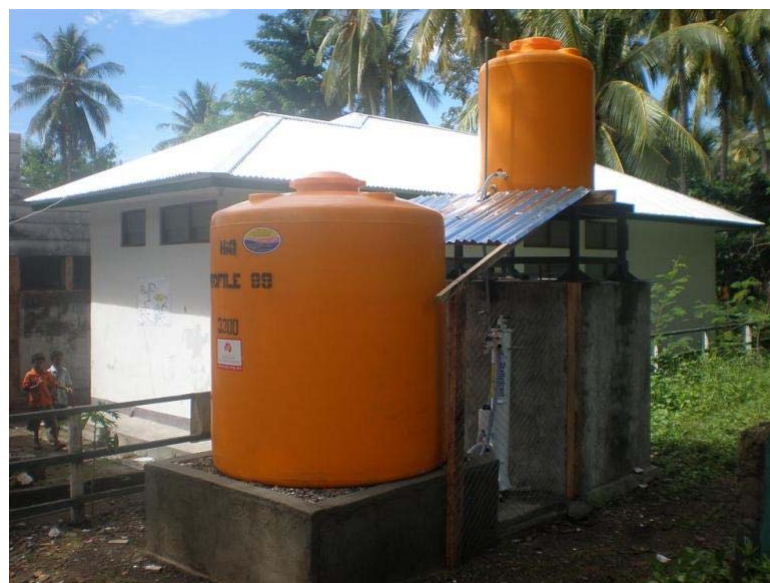
Tank stand and collection tank on the right and tank stand and distribution tank on left
