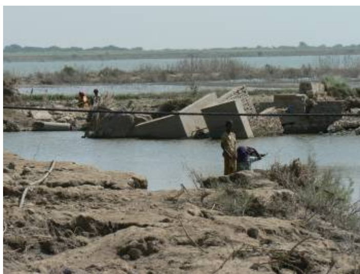
Bridge to Sha Ali Shae village destroyed by the floods reducing access of the local community to services
