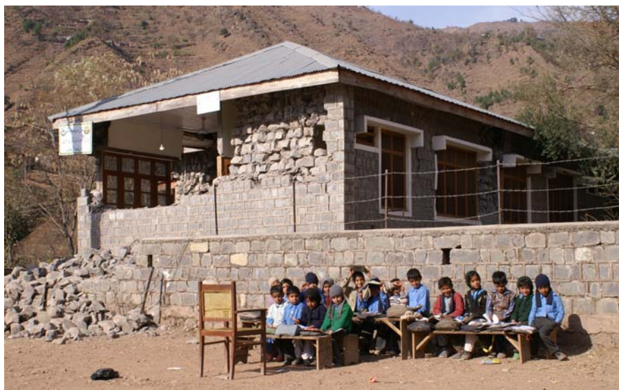
Children attend classes outdoors after their school was heavily damaged by the earthquake.
